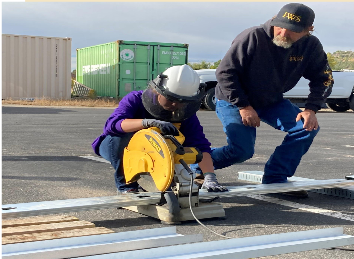
Bayfield student learns how to use a saw during a job shadow with FCI Constructors in October 2021
